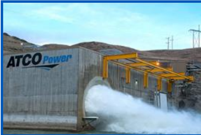
ELECTRICITY GENERATION CANADA 24 MW
