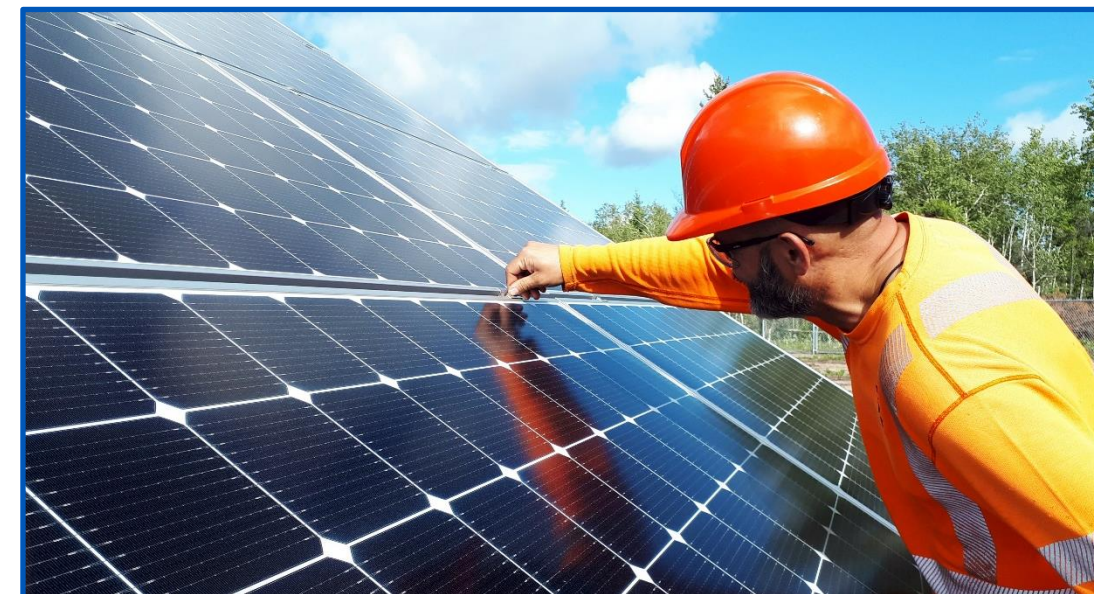
Solar Installation, Fort Chipewyan, AB
