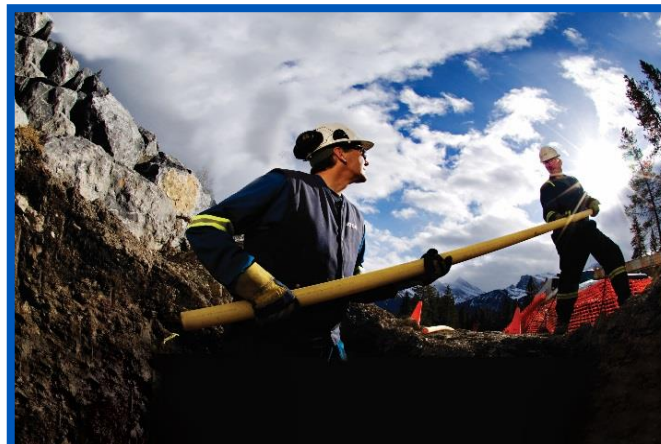
NATURAL GAS DISTRIBUTION $2.9B Rate Base
