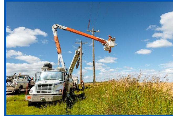
ELECTRICITY DISTRIBUTION $2.6B Rate Base
