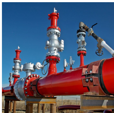
Natural Gas Pipeline Valve Assembly
