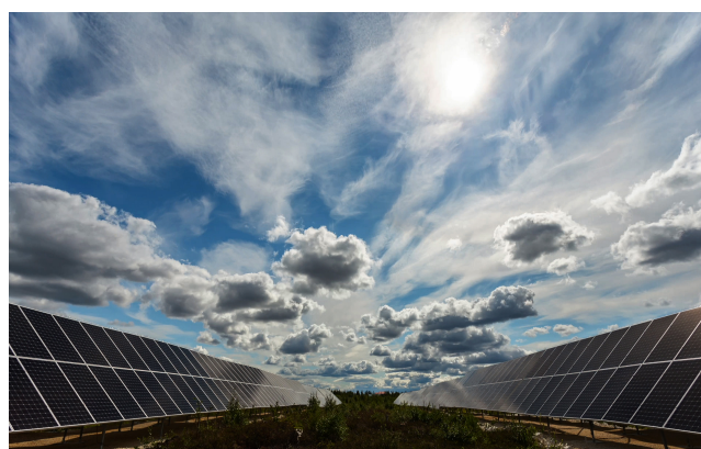
Old Crow Solar Project - Old Crow, Yukon
