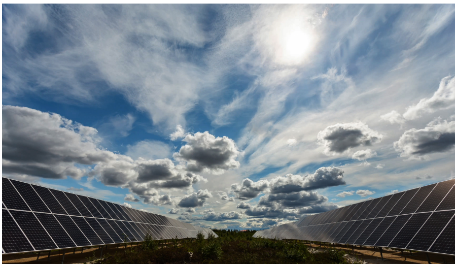
Old Crow Solar Project - Old Crow, Yukon
