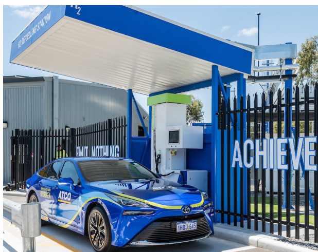
Western Australia's first Hydrogen Refuelling Station
