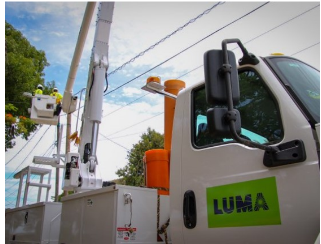
LUMA Energy, Puerto Rico
